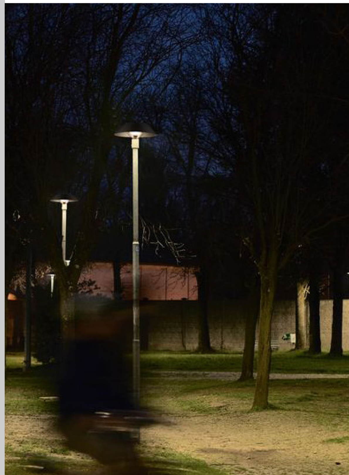
Path lighting at night
