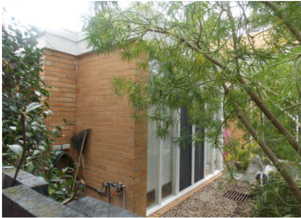
Figure 15: Original part of house at 21 Grandview Grove, Armadale (Kevin Borland, 1955-56) Source: photograph by Built Heritage Pty Ltd
