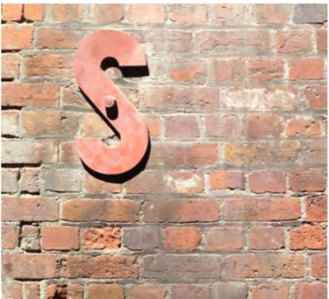
W01: EXISTING BRICK WALLS, STABILISED AND RETAINED. BRICK WALL TO BE RETAINED AND STABILISED WHEN BUILDING IS DEMOLISHED. APPROXIMATE HEIGHT 6m.
