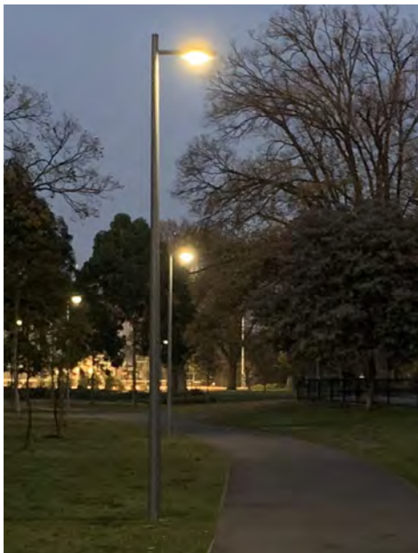
L01: POLE LIGHT, WITH LED LUMINAIRE
