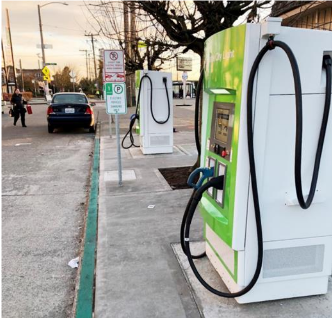
Figure 66 Two DC Fast Chargers owned by Seattle City Light on the 2500 block of 16th Avenue S
