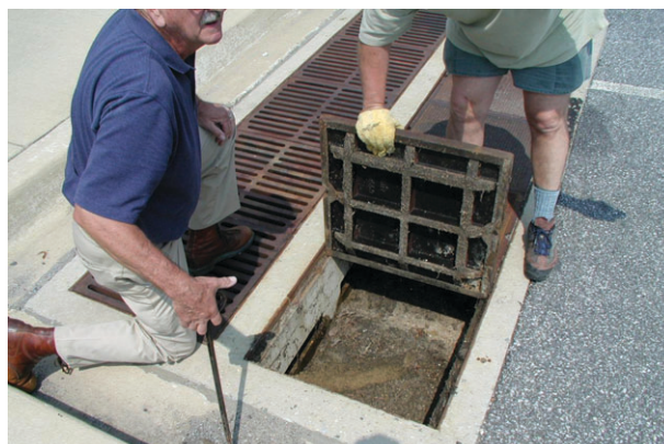
Sand filters for detention and filtration of stormwater runoff
