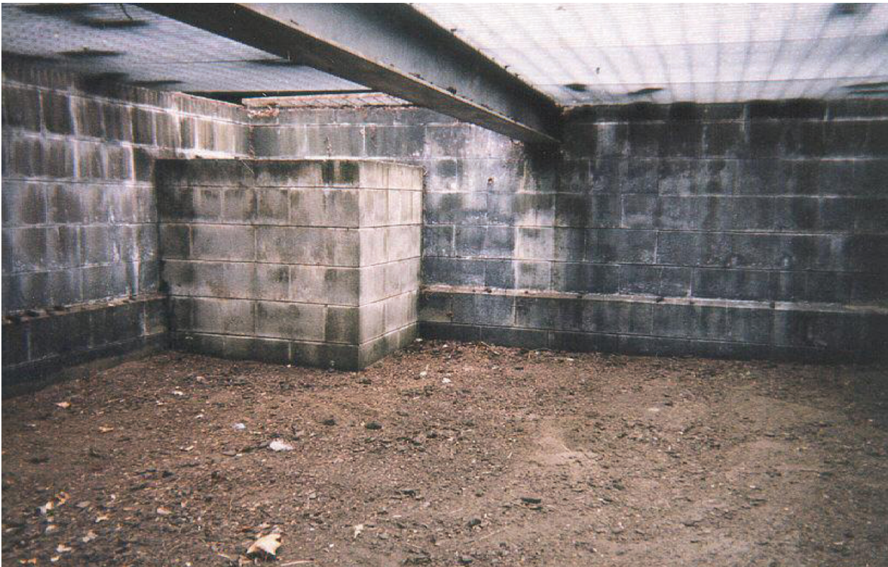
Figure 7.2 Underground sand filter for a car park in Auckland, New Zealand.
