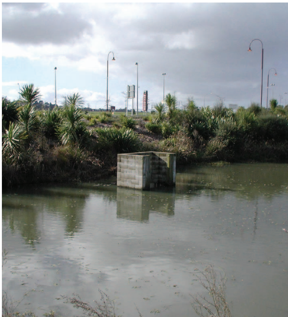
Figure 4.6 Sedimentation basin outlet structures: (a) a floating skimmer and (b) a narrow weir.
