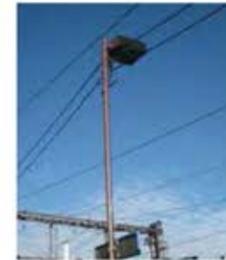
Lighting along station platform
