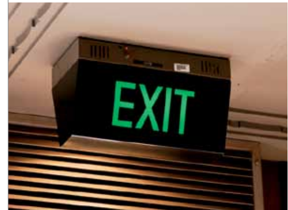
'theatrical' exit signs should be considered in large venues
